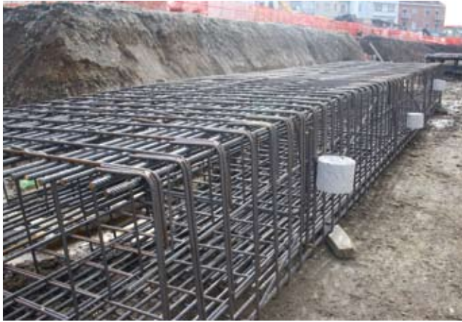
Reinforced cage with spacer to prevent contact between cage and hydromill module in panels overlapping.
