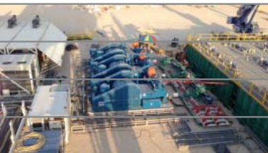
Mud system and Power System.
