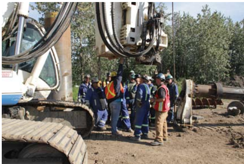
Soilmec and its North American agents team provide week-long training seminars to customers and local union operators.
